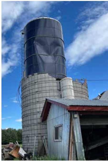
The cement silo was destroyed, damaging the steel silo it stood next to in Rigaud.
